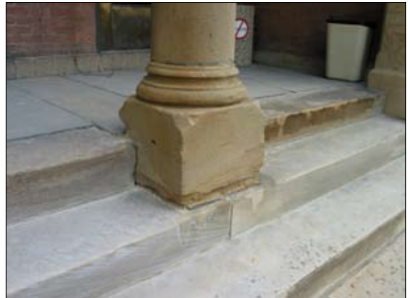
Repair damaged stone to match color and texture.
