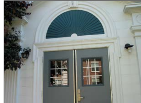
Replace modern fixture with appropriate period light.
