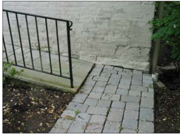
Fix rise to meet ADA requirements.
