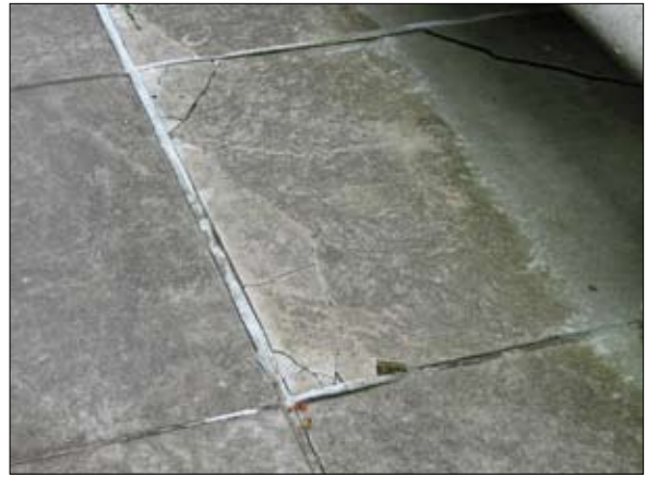
Replace or repair damaged stone pavers as needed.
