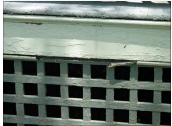
Repair or replace with similar materials.
