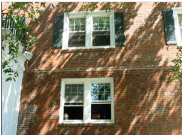
Repoint and match masonry color and texture.
