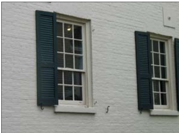
Replace missing shutters.
