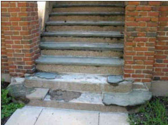
Repair as soon as possible. Liability problem.
