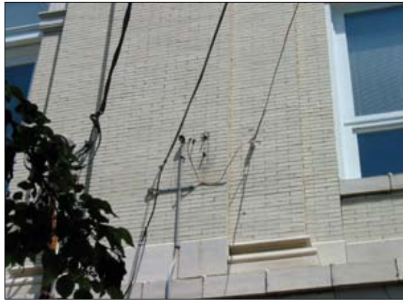
Remove abandoned hardware.
