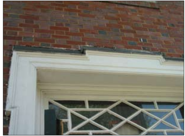
Recaulk fenestrations as needed.
