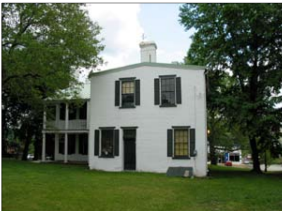
Remove vegetation from chimney.
