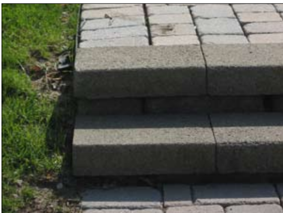
Consider replacing with single-grade walkway.
