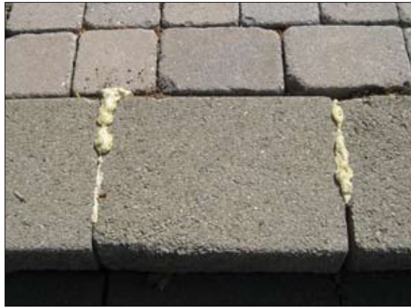
Consider replacing with single-grade walkway.
