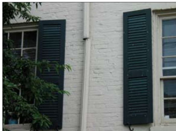
Downspout disconnected. Repair.
