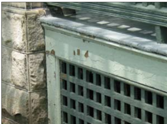
Repair or replace with similar materials.
