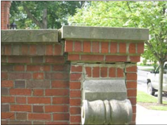
College St. gate damage. Match color and texture.
