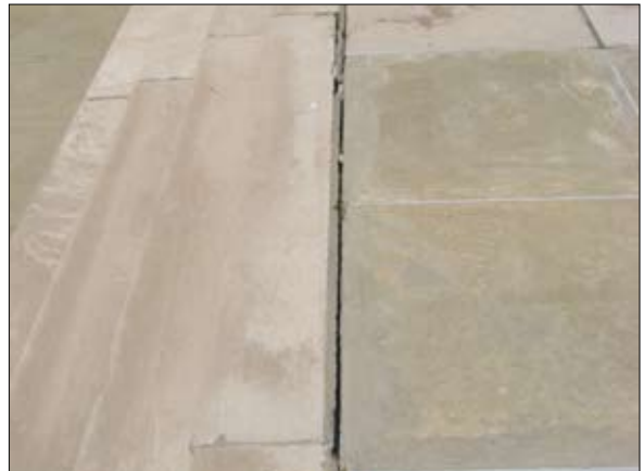
Seal open joints to prevent further damage.
