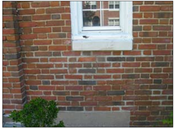
Bad repair. Match color and texture on repairs.
