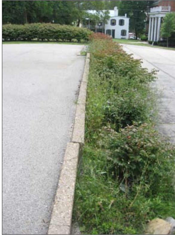
Wall is leaning. Monitor and repair when necessary.
