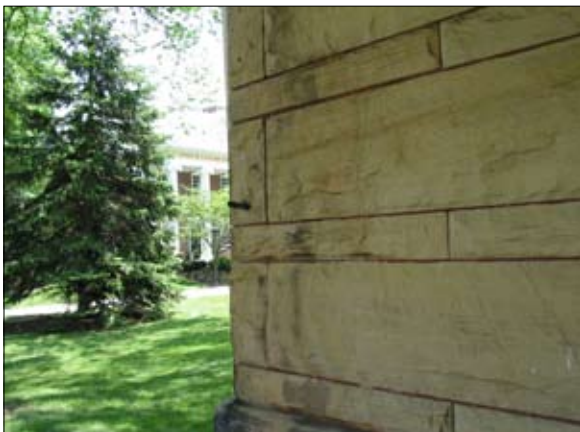
Prune trees back from structures.
