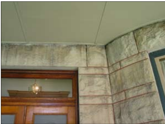
Check roof and flashings. Evidence of water leakage.
