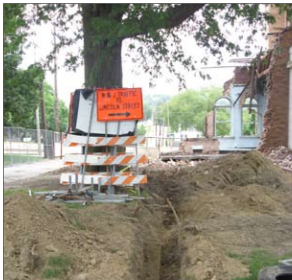
All trees in location of construction should have root aeration after construction is complete.
