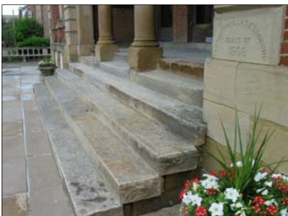
Consider period handrail for safety.
