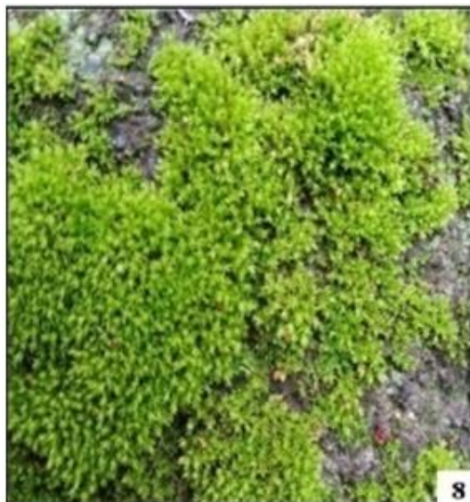
Fig 8: Dominant moss community of Semibarbula orientalis , Hydrogonium amplexifolium , Didymodon recurvus and Hyophila involuta on cementing material of retaining walls.
