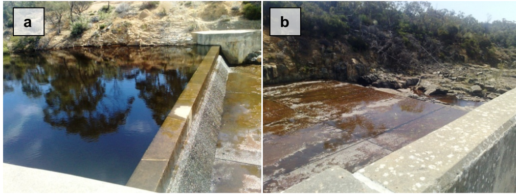
Figure 5. a) Spillway wall step barrier onto concrete apron and b) from apron onto bedrock channel. Picture courtesy of Kumar Savadamuthu (DfW)
