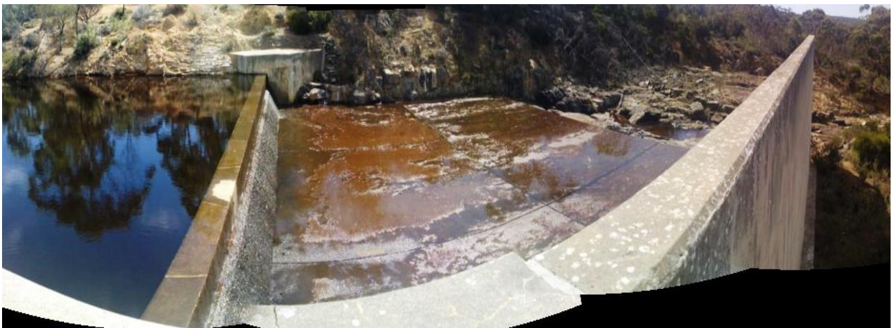
Figure 4. Panorama of the spillway at Middle River reservoir during full reservoir levels. Picture courtesy of Kumar Savadamuthu (DfW)
