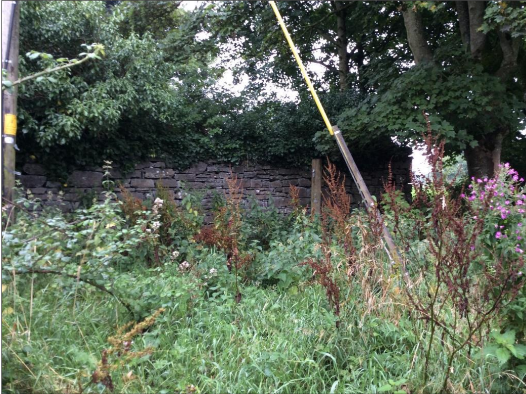
Plate 13-35: Ruinous remains of stone structure at east end of proposed link road.
