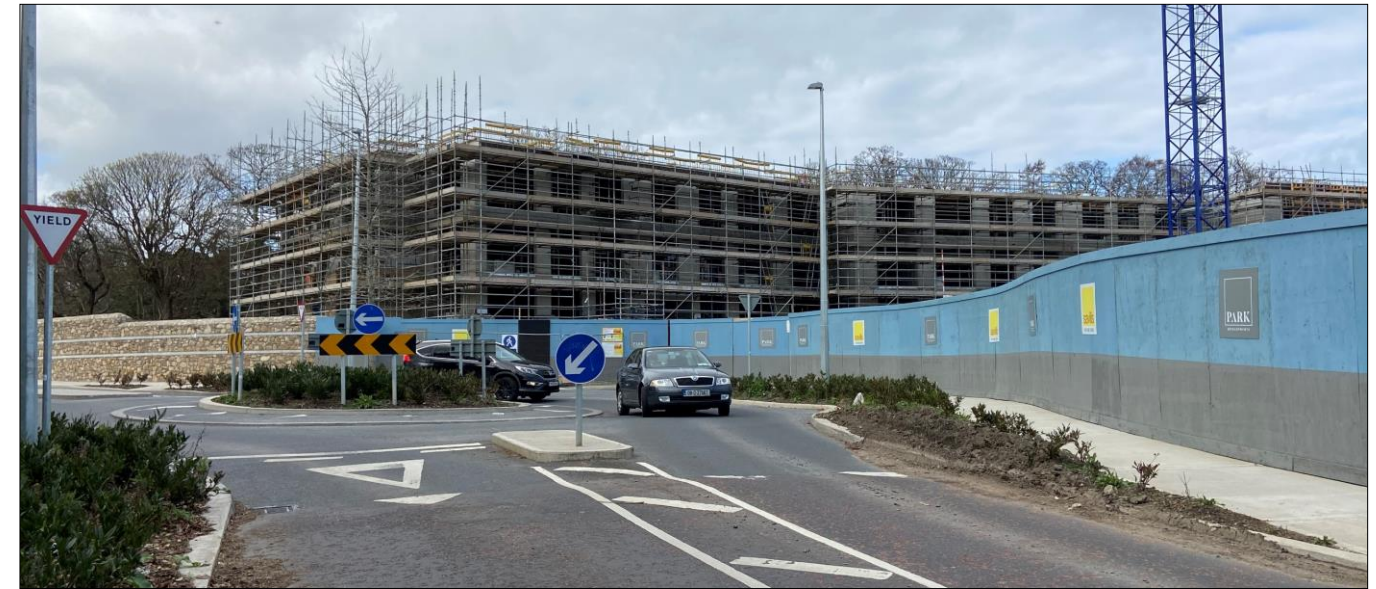
Figure 10.9 The Brennanstown Wood development under construction in 2021, c. 150m from the site. This illustrates the change in character taking place along Brennanstown Road in the vicinity of the site
