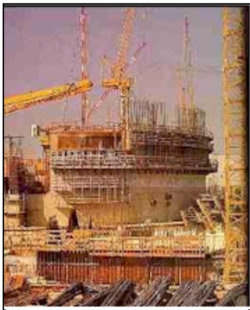
Bushehr Nuclear Power Plant
