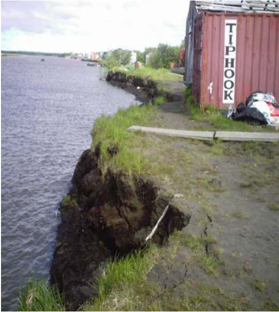
Photo 1: Bank erosion along the Kotlik shoreline, 2007.
