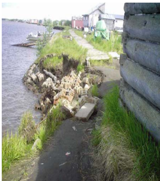
Photo 4: Concrete blocks, remnants of failed erosion protection litter the shoreline, 2007.
