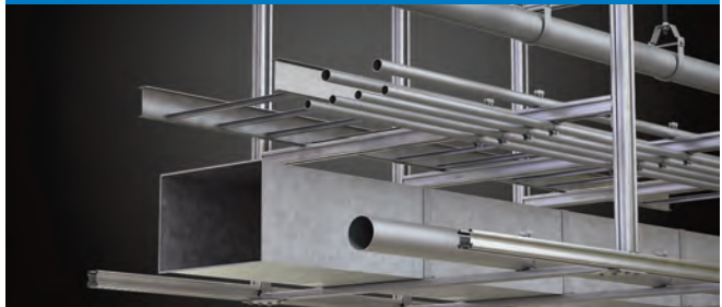
Overhead racking application
