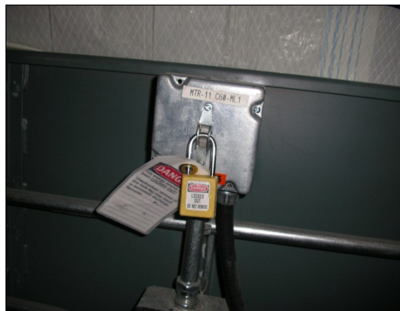
LO/TO AT UPSTREAM DISCONNECT (I.E. MOTOR #11)
