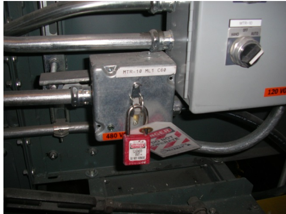
LO/TO AT THE LOCAL DISCONNECT (I.E. MOTOR #10)
