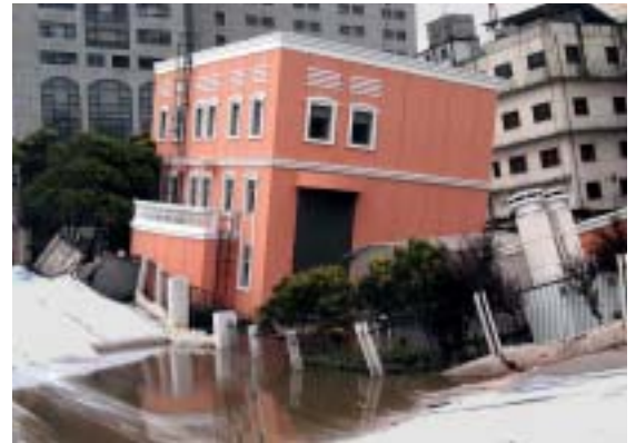
1 July 2003, Shanghai, People's Republic of China: Subsidence had a devastating effect on buildings after a massive influx of material and water into a cross passage under the Huangpu River.
