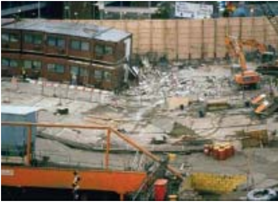
21 October 1994, London, UK: There was considerable surface subsidence in three of the headings for the Heathrow Express Link, finally leading to the tunnels caving in.
