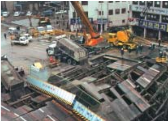
22 January 2000, Taegu, South Korea: Following the failure of a diaphragm wall, part of an underground station excavation pit caved in. The consequences? A whole section of road gave way and cracks formed in buildings.
