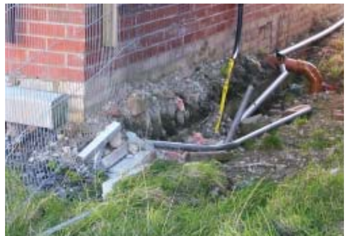
Drains, water pipes, gas pipes, and power lines shifted and cracked.
