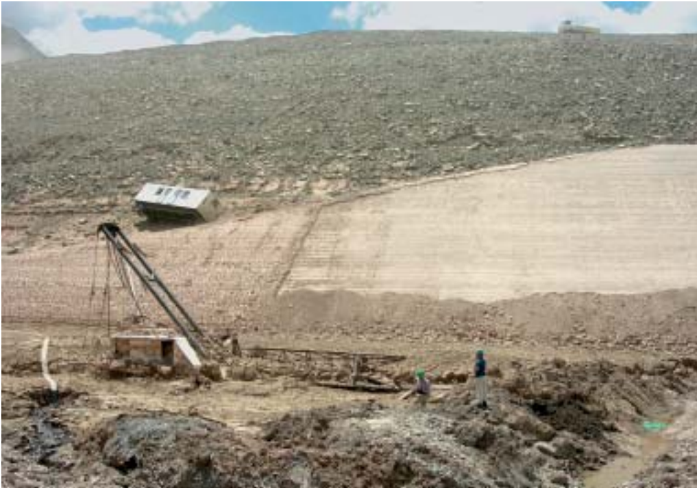
A still partially buried crane in front of the main dam. As the machines used in dam construction are technically sophisticated and expensive, the loss is enormous in most cases.
