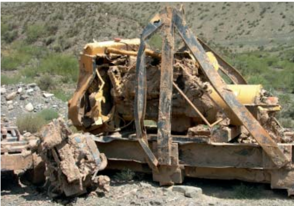
The remains of a diesel generator – completely deformed by the strong flow of water and debris.
