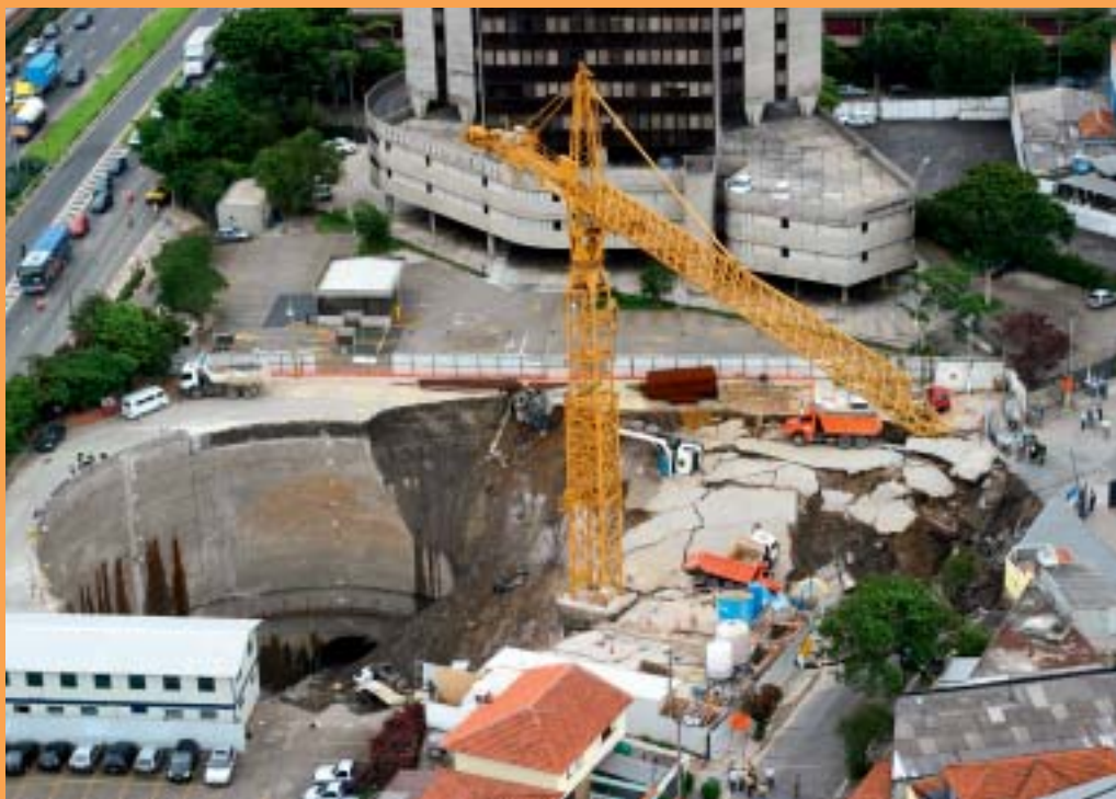
12 February 2007, São Paulo, Brazil: The launching shaft and parts of the running tunnels beyond collapsed during work on a new underground station.
