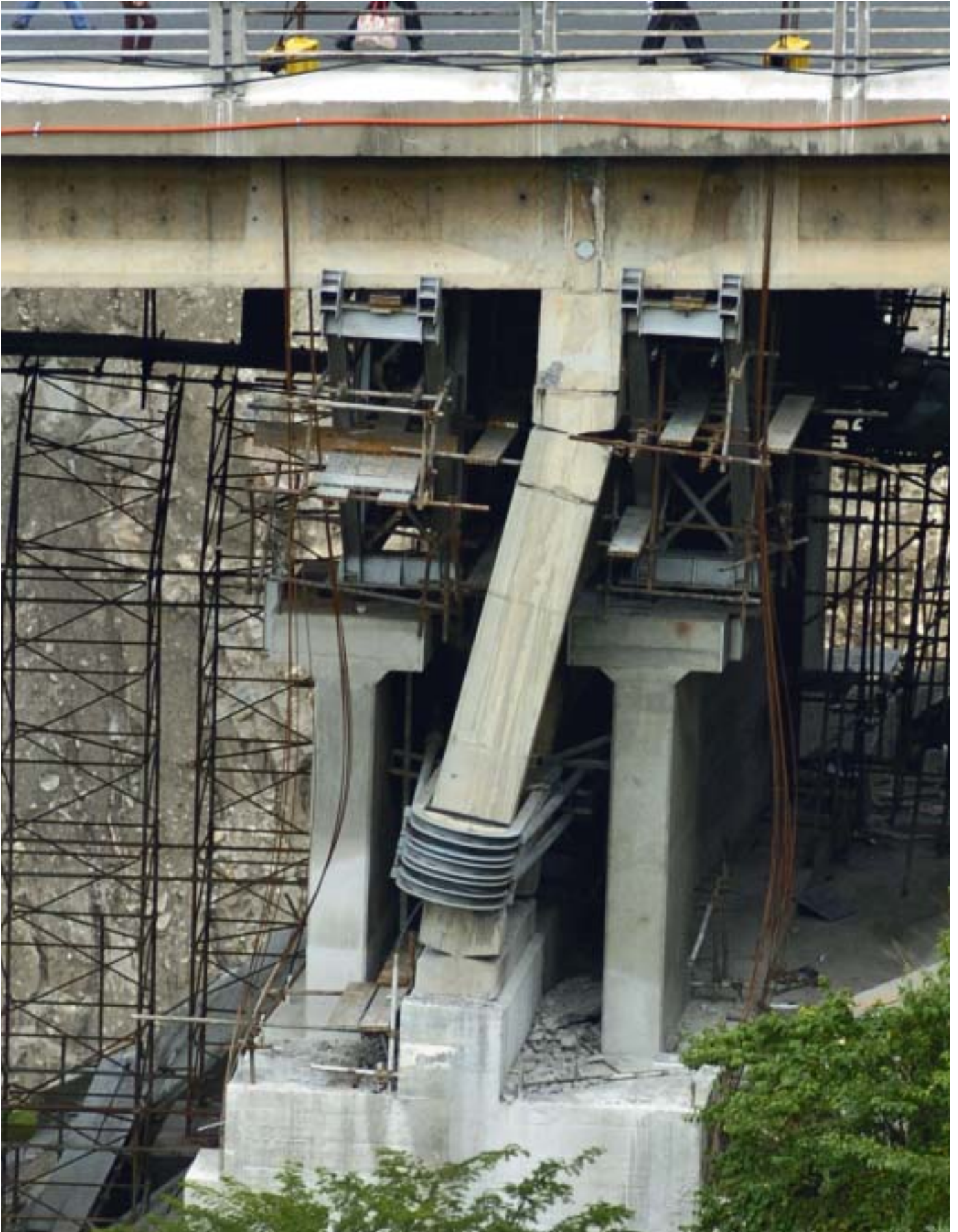
... but nothing could be done to avert the collapse.
