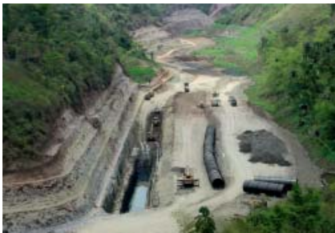
The pipeline had to be re-laid. One of the design improvements: replacement with a pipe with thicker walls.
