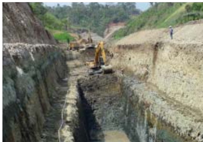
A further improvement: the trench was reinforced with concrete on the slope side, thus reducing the pressure on the new pipeline.
