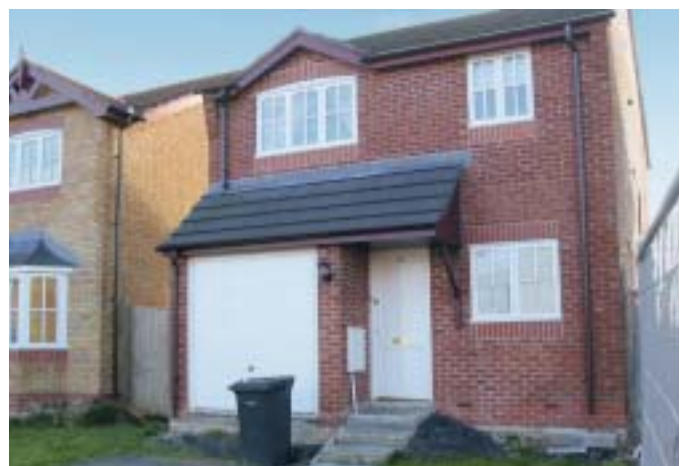
Phase 2 house, constructed on pile foundations. The surrounding ground became compacted, however, and subsided.
