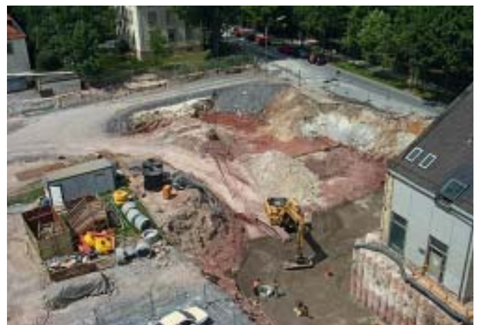
The remediation plan implemented in 2000 included a large-scale excavation of the soil down to a depth of 5 m – not the most favourable solution in either economic or ecological terms.
