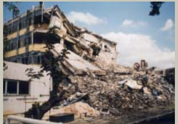
Athens, Greece, 7 September 1999. Here too, much of the damage could have been avoided by paying attention to good construction work and observing the regulations.
