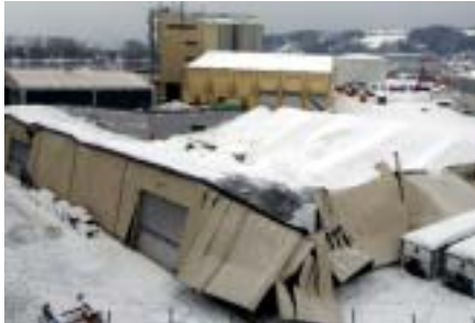
January–March, Europe Winter damage
