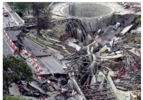
20 April 2004, Singapore: A retaining wall for the Circle Line collapsed, resulting in severe damage to the six-lane Nicoll Highway directly beside it.
