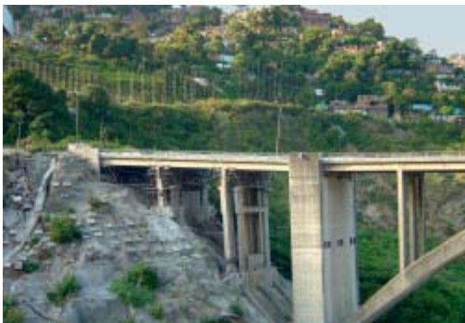
Viaducto Uno at the beginning of 2006: the piers were still supported by scaffolding ...
