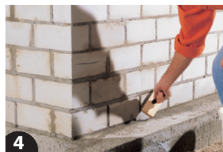
4 In the next step a concave fillet is then formed along the wall/floor contact. The site is wetted with a brush for better adhesion of the mortar.
