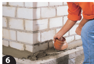
6 A plastic pipe or similar can be used to create the concave fillet. This produces a rounded transition from the wall to the floor slab.
