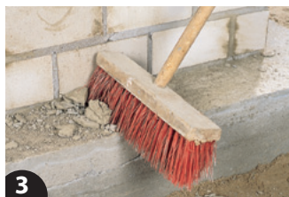
3 The loose mortar residues are then swept with a broom from the floor slab.
