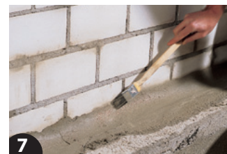
7 At the transitions between the mortar and the substrate, the interface is to be smoothed with a damp brush.
