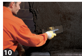
10 The thick coating is applied with the trowel in two layers on the substrate. Depending on the load, the coating must have a wet film thickness of at least 4 or 6 mm. The result is a seamless water-proofing layer.
