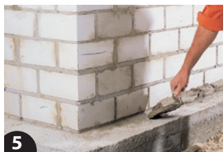
5 PROBAU Cement Mortar is applied with a trowel in individual dabs of mortar on the floor slab.
