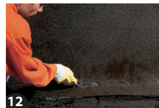
12 Finally, the concave fillet is again smoothed with a tongue trowel. After thorough drying of the thick coating, perimeter insulation boards are bonded to protect the seal. Only then can the filling up of the work area commence.
