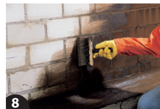
8 In the next step, the exterior basement wall is coated with a solvent-free primer. For this, PROBAU Thick Bitumen Coating is diluted 1:10 with water and applied with a brush to the entire surface of the area to be treated.
