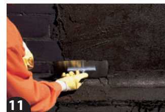
11 The thick coating is also applied evenly in the concave fillet, so no leaks can occur here.
