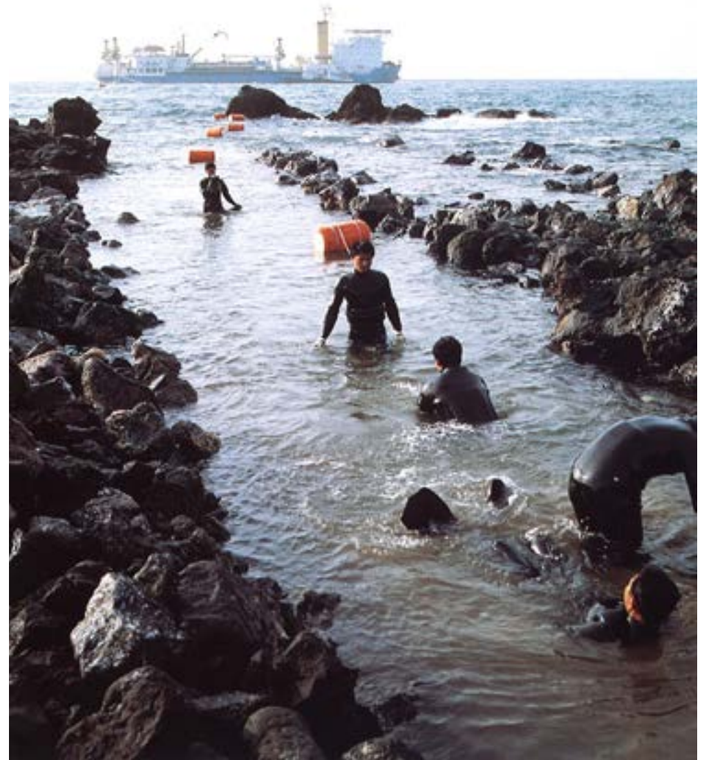
Divers pulling submarine cable ashore with the cableship Giulio Verne in the background.
