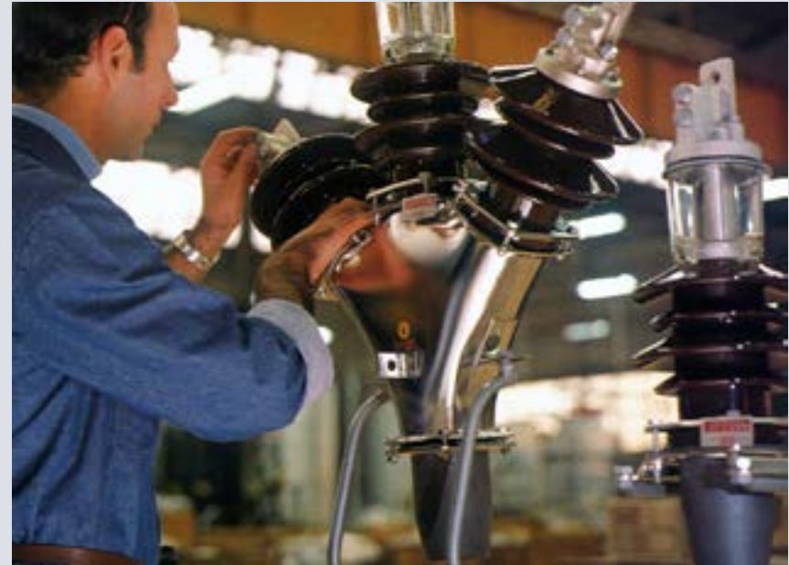
Three-core medium voltage terminations, with insulant level sight-glass.
