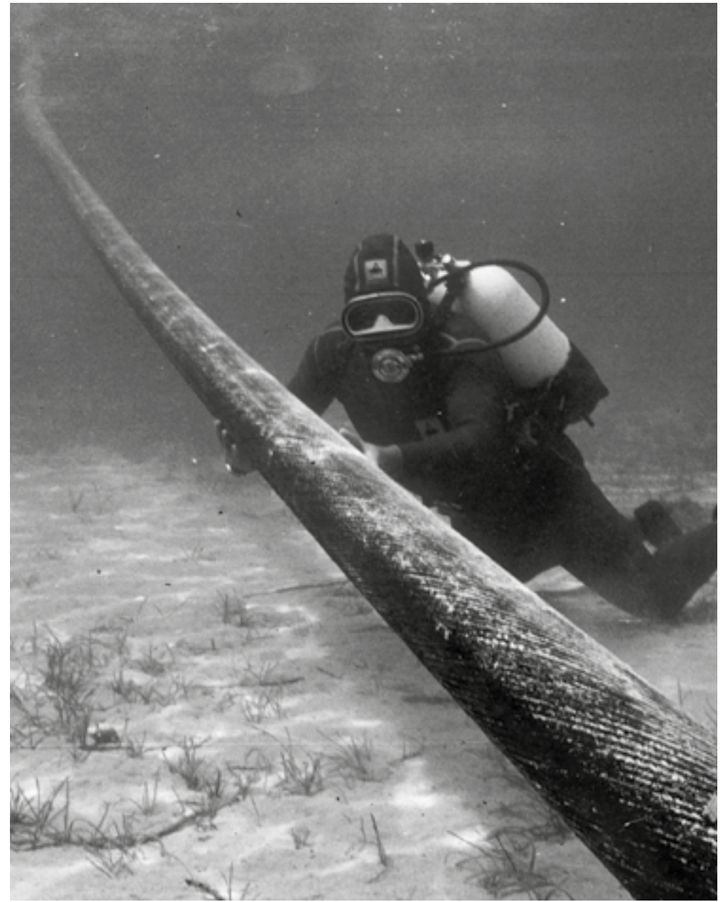
6 th December 1971, a frogman in scuba gear at work in the Mediterranean Sea during the laying of freshwater pipelines between mainland Sardinia and the offshore island of San Pietro.
