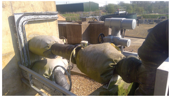
Figure 2.1 Poorly installed flow to full treatment flow meter
