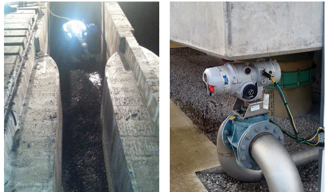
Figure 2.2 A large flume influenced by poor maintenance procedures allowing grit build up
