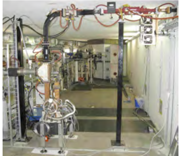
Figure 4: The CTF gun number 5 in the SLS linac bunker during the high gradient tests.
