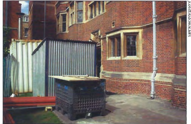
The temporary boiler house serving Docket Building over the summer.
