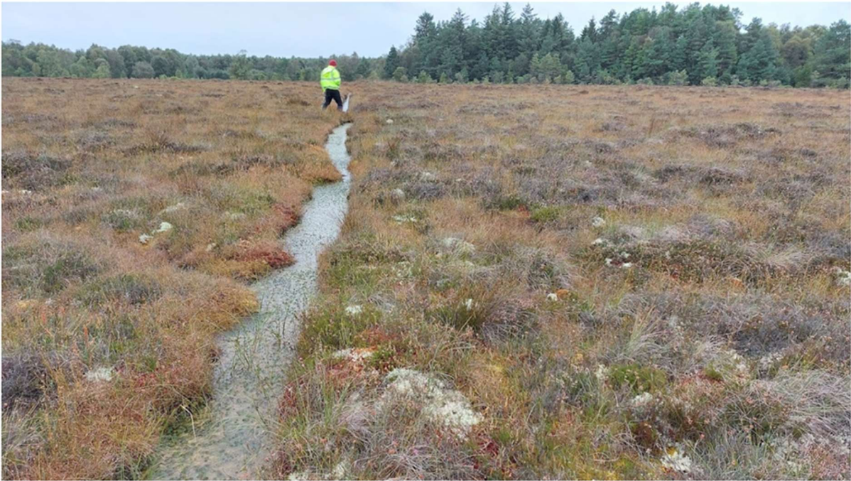
Figure 5.5 High Bog Drain in Lough Forbes to be staked out and blocked
