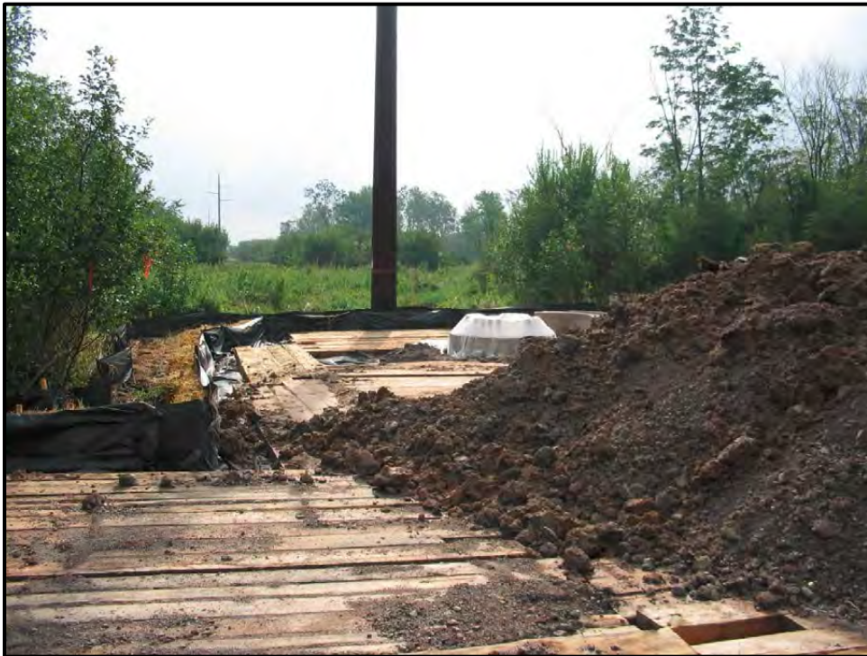
Figure 2.4-11. Structure location in a wetland—matted work platform, foundation, spoil pile (to be removed), and erosion control.
