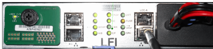
Figure 1-44 Library frame interconnect
