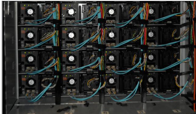
Figure 1-32 TS4500 drive bay
