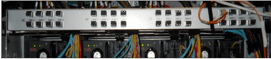
Figure 1-46 Fiber patch panel
