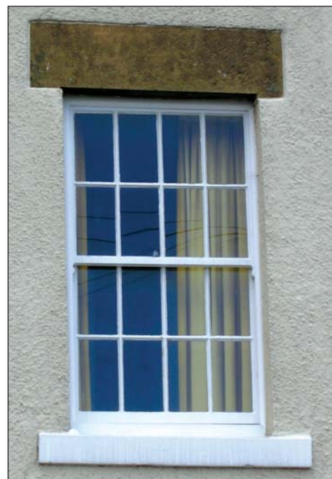
Picture 6. Traditional wood, vertically-sliding sash window with stone lintel and painted sill
