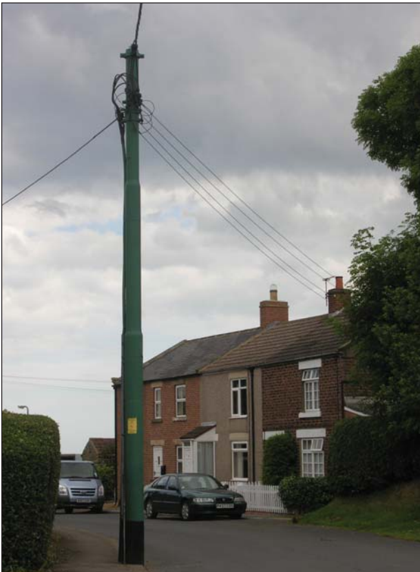
Picture 34. Unsightly electricity distribution pole
