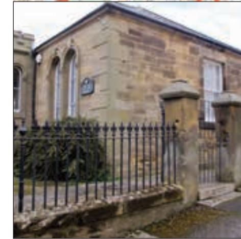
Boundary/Retaining Wall, Railings and Gatepiers to Front Yard of The Old Zetland School. Grade II - 1136477
