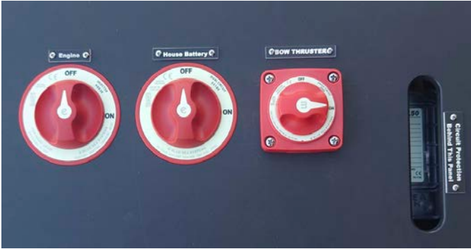
Photo: Battery Management Box with “Engine”, “House Battery”, and “Bow Thruster” switches.
