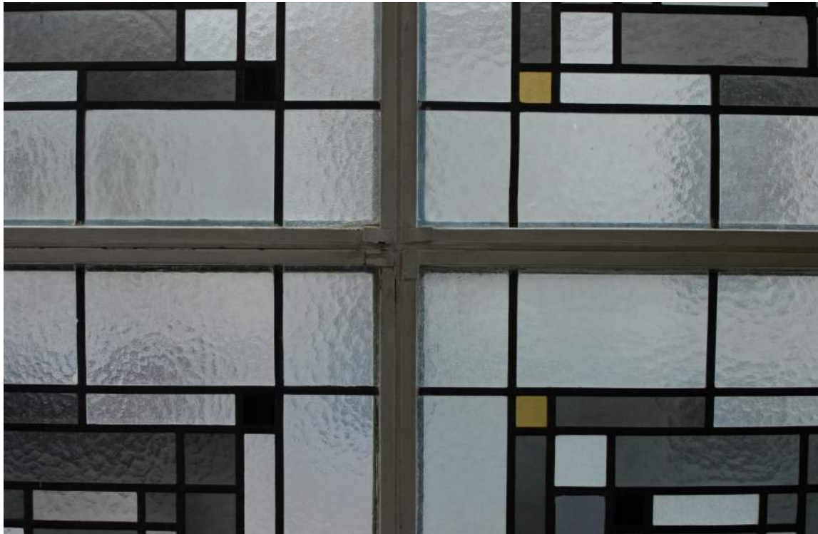
Detail of glass stop tabs, steel window at St Hedwig. Photo by author.
