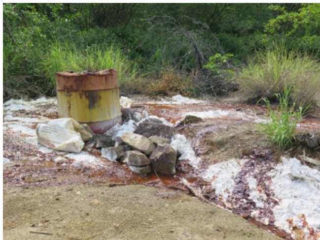
Suppl.-Figure 27 Plugged former service borehole, AMD effluent reaches the surface. Picture taken 21.03.2018 at 18°20'14.96"S, 26°29'7.04"E
