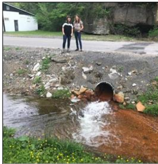
Mine drainage into Sandlick Creek downstream of the Fire Department.
