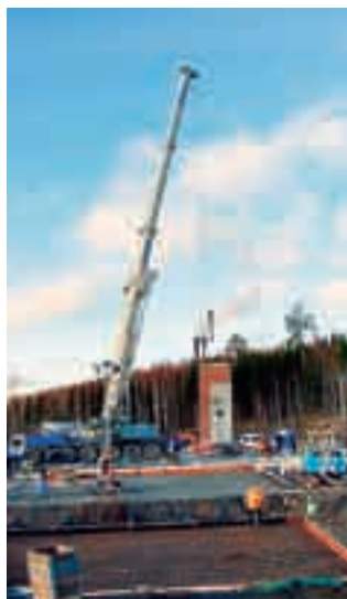
The construction of a new effluent treatment plant at Iggesunds Bruk began in the autumn.
