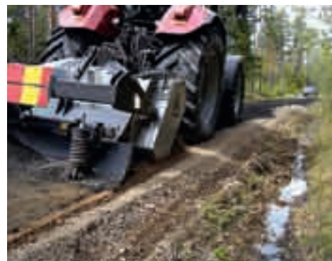
A mixture of ash and green liquor sludge from Iggesunds Bruk undergoing tests as the roadbed on a forest road.
