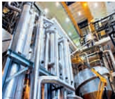
The new energy-effective pulp line at Braviken.
