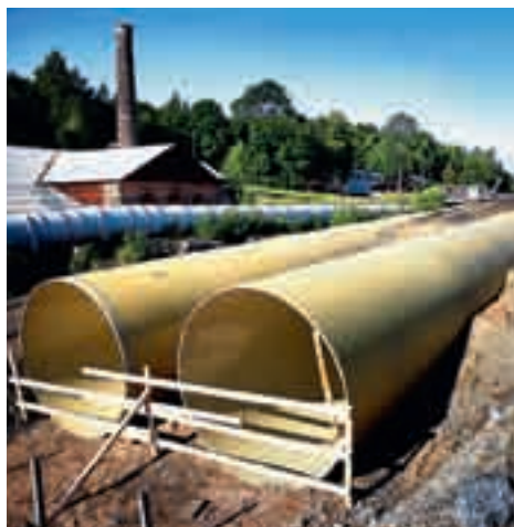
A new hydro power plant is being constructed at Iggesund to replace three old ones.
