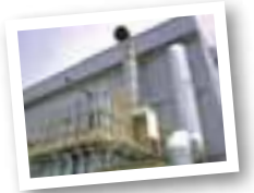
Using exhaust heat
