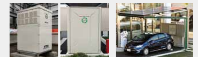
Smart Green Batteries recycling end-of-life Prius batteries
