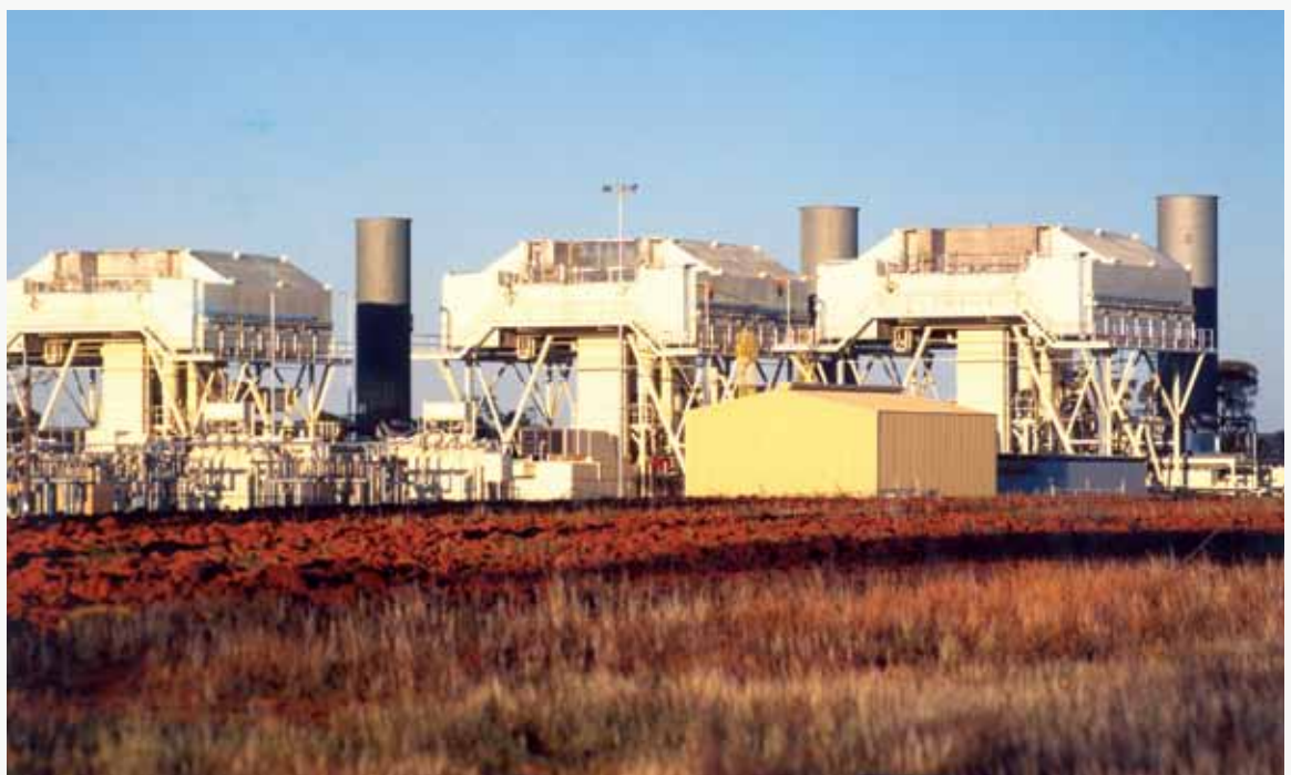
Parkeston gas-cogeneration plant in Western Australia.
