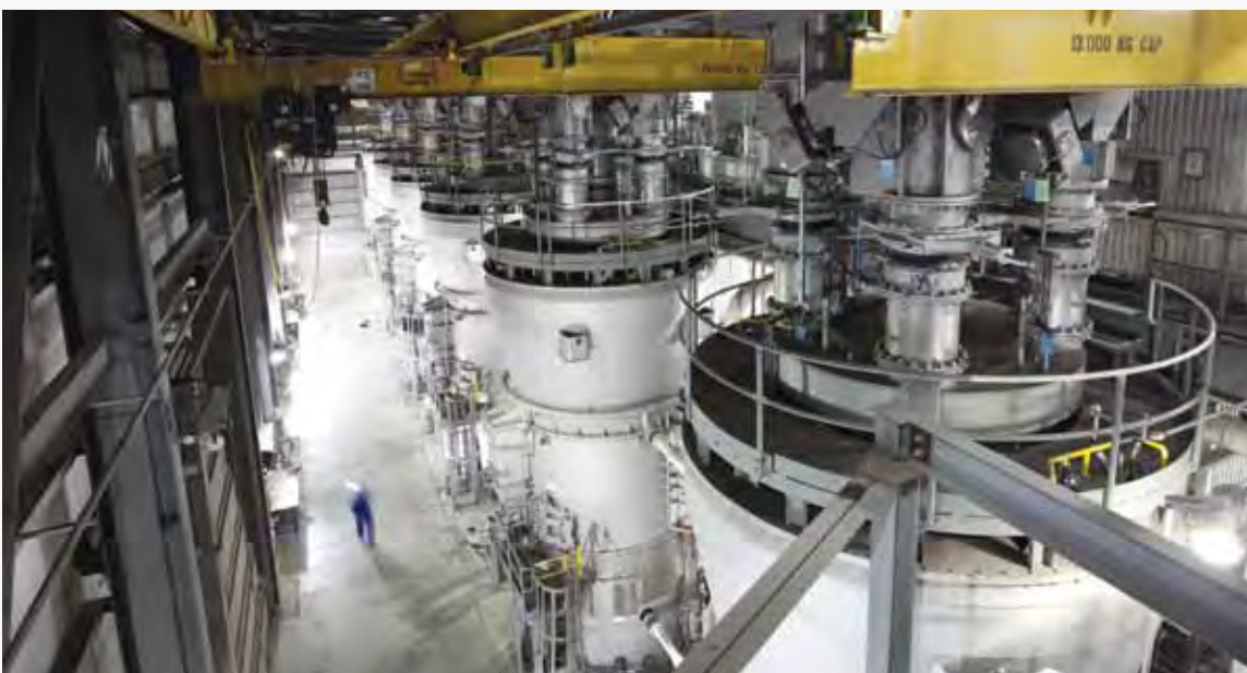
The gleaming coal pulverizers or coal mills (six in total) at Keephills 3 which pulverize the coal to a fine powder before it is blown into the boiler.
