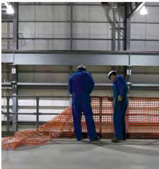
Workers install safety netting to prevent falling objects and improve workplace safety.
