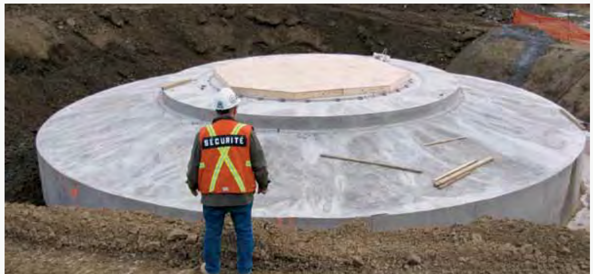
At the time of this report’s production, 23 of the 33 cement turbine foundations had been poured for the New Richmond wind facility.
