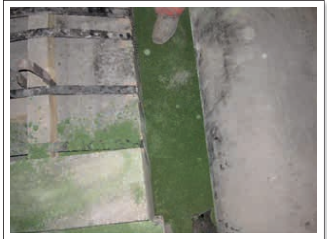
Figure 6. The remaining gaps towards the breast electrode and steel shell were rammed with ANKERMIX NP13.
