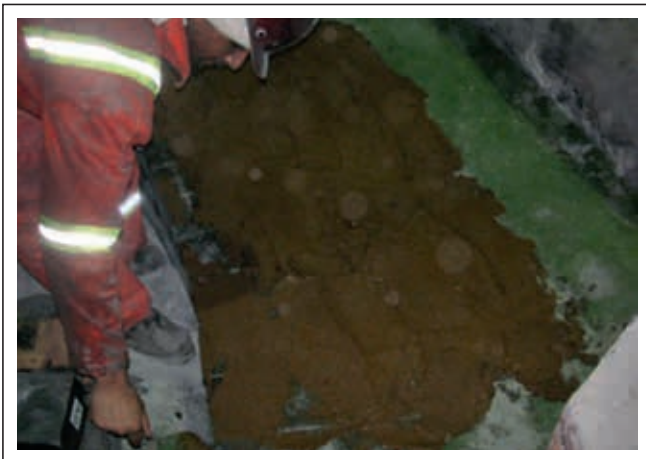
Figure 4. An overhead crane was used to maneuver the block into its final position. A 10-mm ANKERFIX NS60 (mortar) layer was applied to ensure correct installation regarding levelling.
