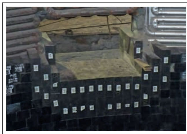
Figure 2. Standard slag door lining. Normally the slag door area is bricked using SYNCARBON C F6T14, a carbon-bonded grade based on medium-quality fused magnesia with a carbon content of 14 wt.%.
