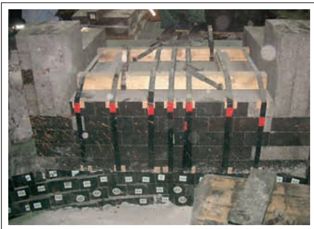
Figure 5. Final placement of the preassembled slag door. Slight modifications to the geometry were required so the cooling panel fitted after positioning the upper split shell.
