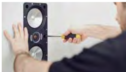
We've big stocks in-store for you to take home today and will gladly advise on installation.
