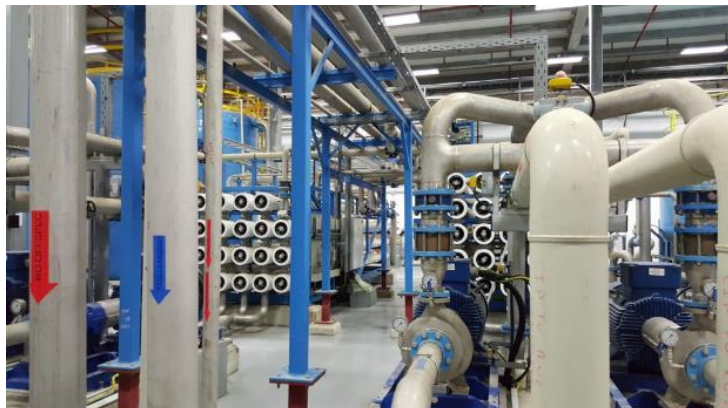
Water treatment hall at the Ashkelon Dorad Electric Power Plant
