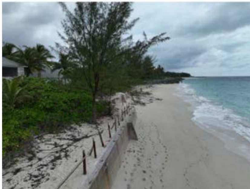
Photo 3-10: Eastern sandy shoreline profile with no vegetation and retaining wall (view facing West)
