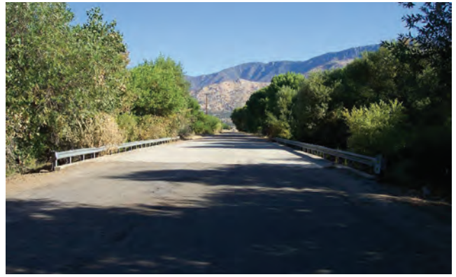
6: Fay Ranch Road at the bridge on the South Fork Kern River
