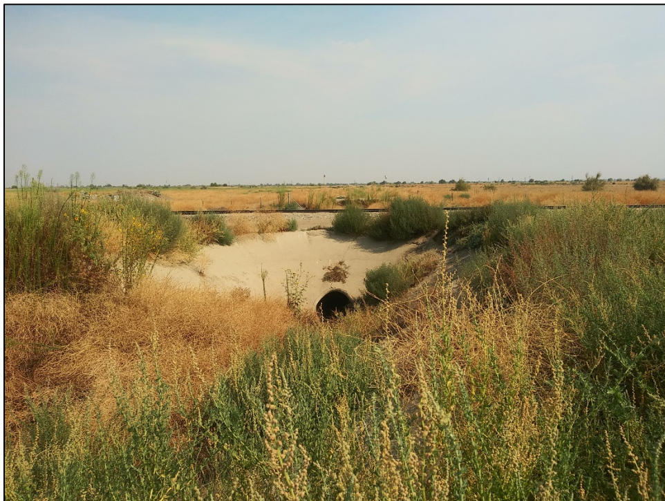
Photo C-12. North view from PP-12 of “James Canal” that passes under railway through culvert (August 18, 2020).
