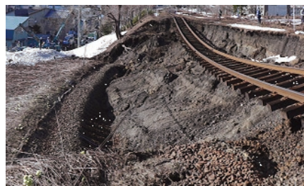
Fig. 2 Example of embankment collapse triggered by infiltration of snowmelt
