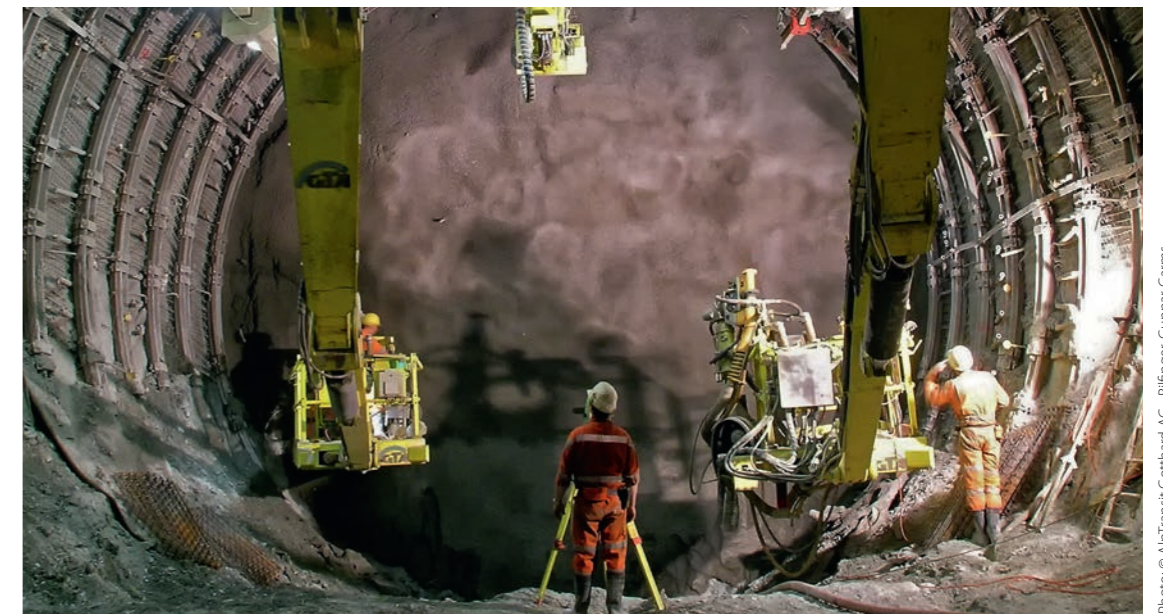
The steel skeleton of the mine support sections during the tunnel construction. It can be very clearly seen how the sections mesh and are held together by the connection pieces
