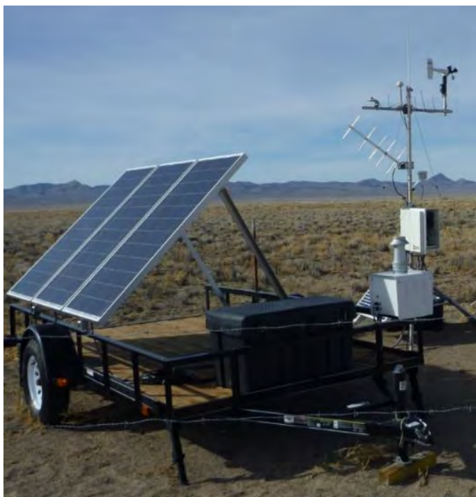
Figure A-4. Station 404, located along the north fence that bounds the Clean Slate II contamination area, includes a solar-powered air sampler and meteorological tower
