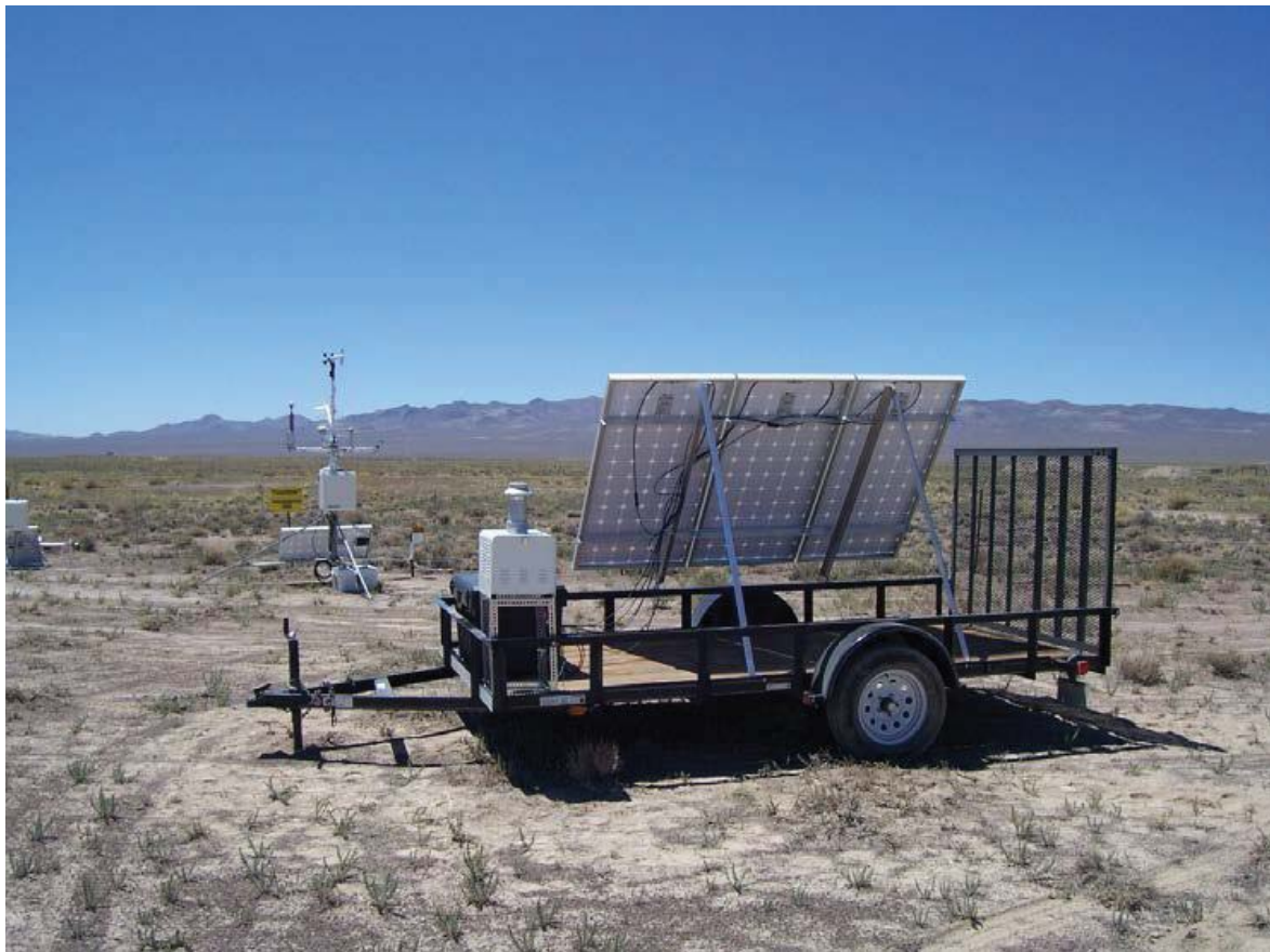
FIGURE 1-6. Station 402 consists of a trailer mounted solar powered air sampler and a portable meteorological tower located on the north fenceline at Clean Slate 1.
