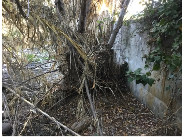
Upstream portion of Reach 2 viewing north-east at the channel left bank (viewing downstream) and vegetation. Note the sediment deposition of approximately 1-foot.
