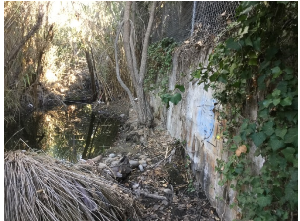
Reach 2 viewing north-east at the channel left bank, concrete wall (viewing downstream), arundo and standing water along the channel bottom.
