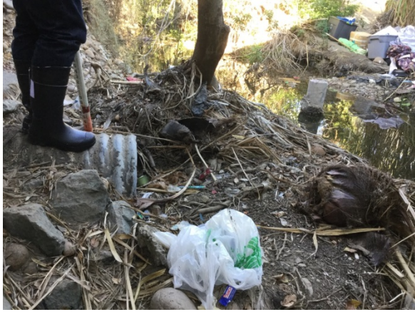
Clogged outfall at the downstream end of Reach 2.
