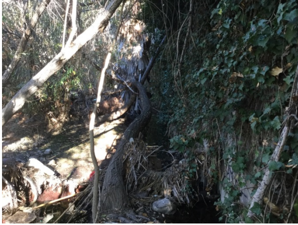
Reach 2 viewing north-east at the channel left bank, concrete wall (viewing downstream) and channel bottom.
