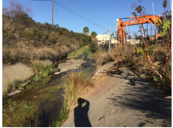
Upstream portion of Reach 3 viewing north-east at the transition in channel geometry from trapezoidal to rectangular.
