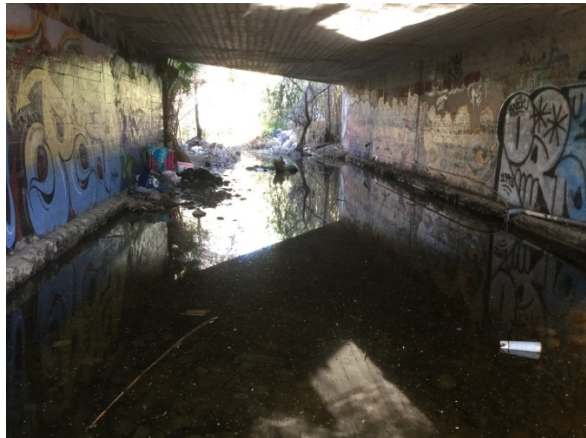
Downstream portion of Reach 2 viewing north-east underneath the bridge at Federal Boulevard. Please note the scour along the abutments.
