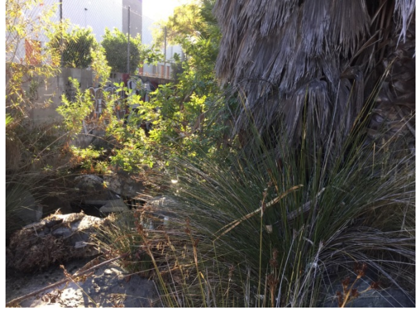
Upstream portion of Reach 2 viewing south-west at the 2-ton rip-rap channel lining and vegetation within the channel (palm trees and arundo)
