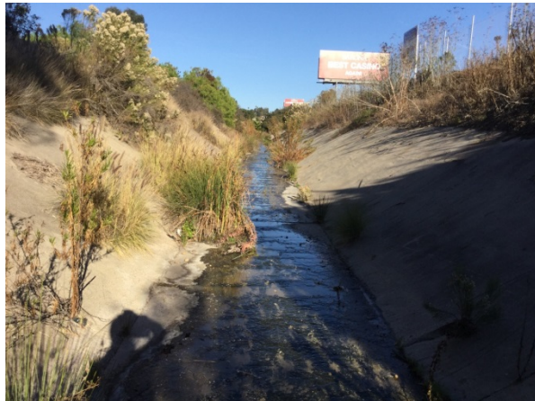
Downstream portion of Reach 3 viewing north-east at the concrete lined channel. Note the minimal vegetation established within the channel.
