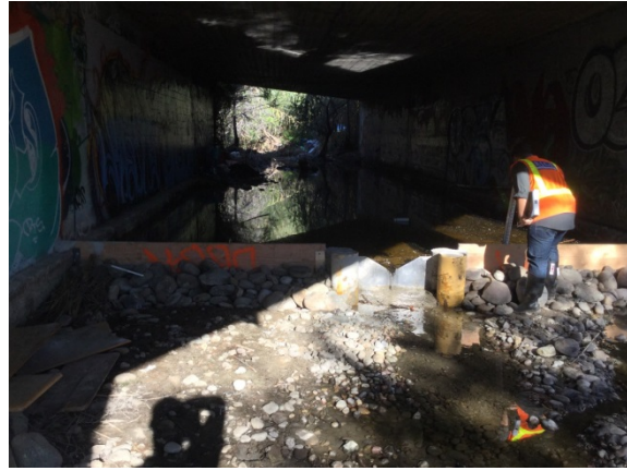
Upstream portion of Reach 1 viewing north-east underneath the bridge at Federal Boulevard (please note the v-notch weir flow indicator).
