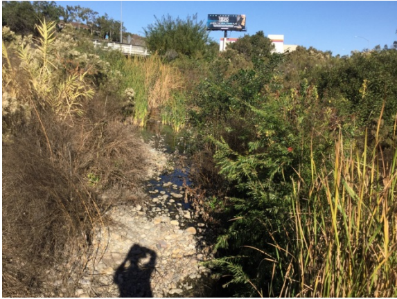
Downstream portion of Reach 1 viewing north-east at the channel and downstream end of the single span bridge at Federal Boulevard.
