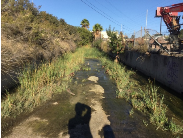
Upstream portion of Reach 3 viewing north-east at the rectangular concrete channel. Not minimal vegetation established in channel.
