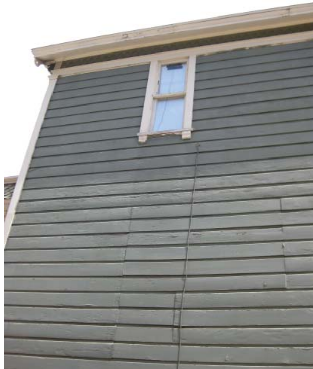
Figure 3-17: The Daggett Family Residence's only remaining historic window located at the second floor of the south facade. All other windows have been replaced.
