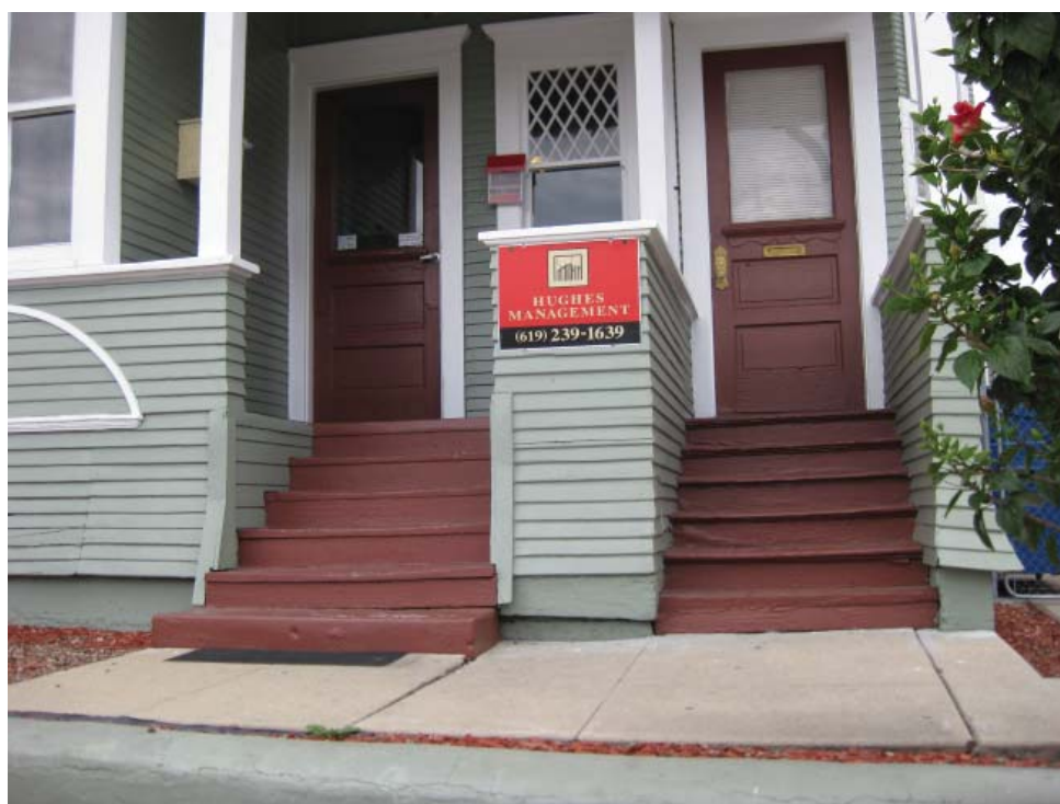
Figure 3-7: The Murray Apartments, view of the front steps on the west facade. The stairs on the right appear to be original. The stairs on the left appear to have been altered to replace the original treads and risers. The front doors and window are original. The door hardware on the right door also appears to be historic.
