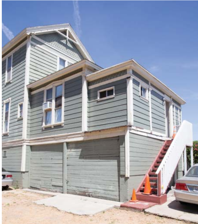
Figure 3-15: The Daggett Family Residence, view of portions of the east and south facades. The former porch (in the foreground) has been filled in to add an additional apartment unit. The garages beneath were added below the original house, raising the house above its original height.
