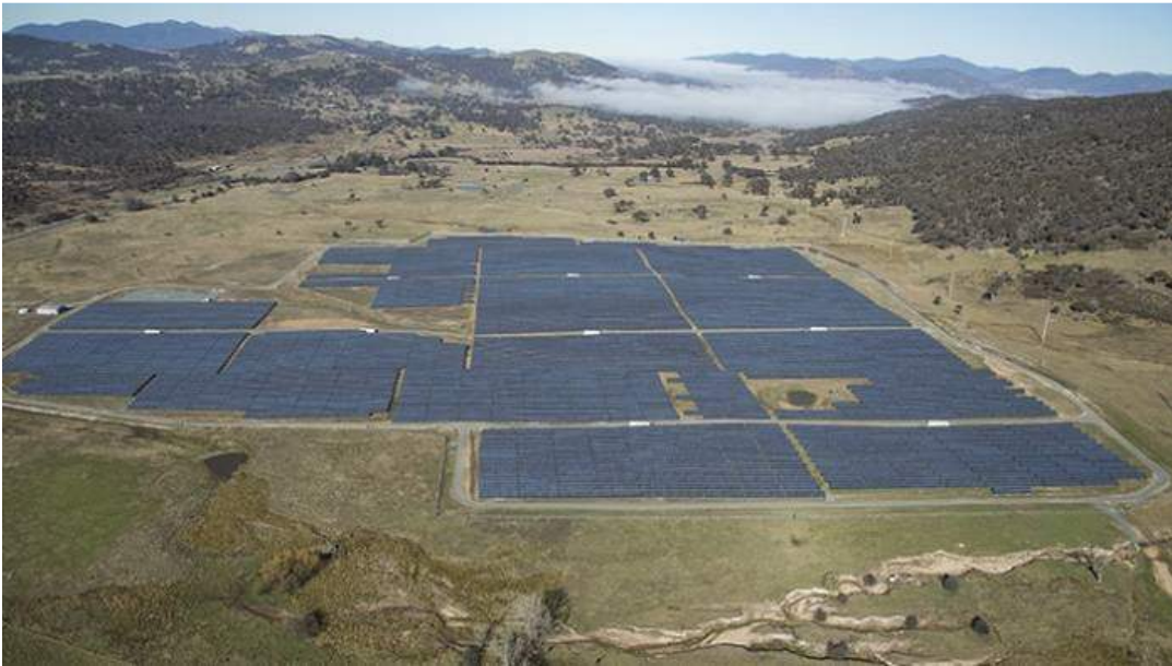
Solar: Royalla Solar Farm (ACT). Photo: royallasolarfarm.com.au
