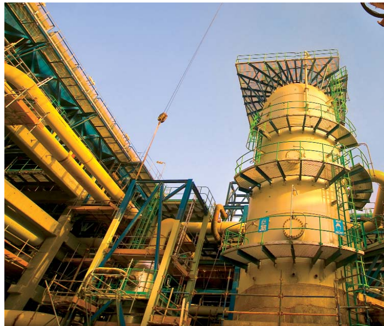
The Oryx GTL plant in Qatar will supply environmentally preferred synthetic diesel.
