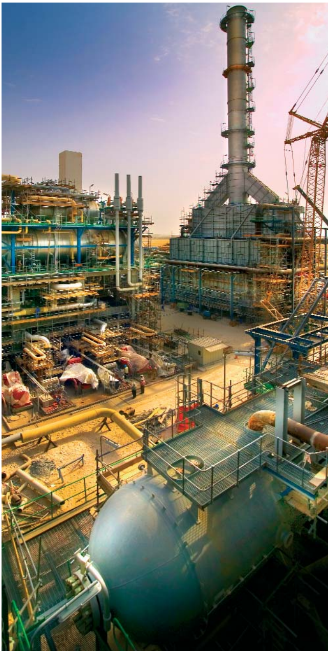
The Oryx GTL plant in Qatar will be brought into production in the year ahead.
