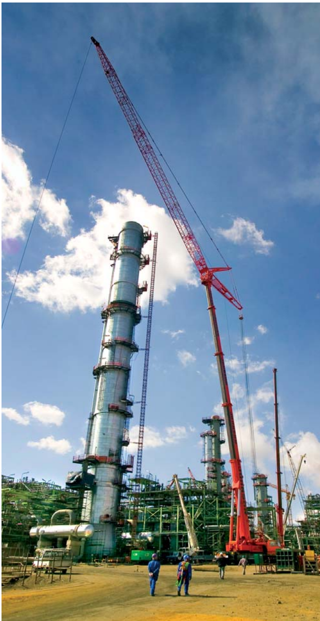
Project Turbo work in progress under the vigilant eyes of Sasol Technology engineers and project managers.
