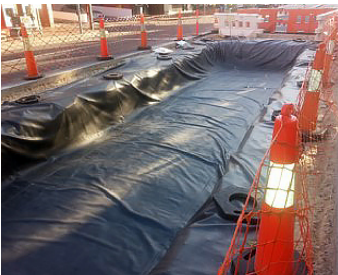
Poly membrane liner being laid at the base of tree pit to protect underground wastewater pipes.
