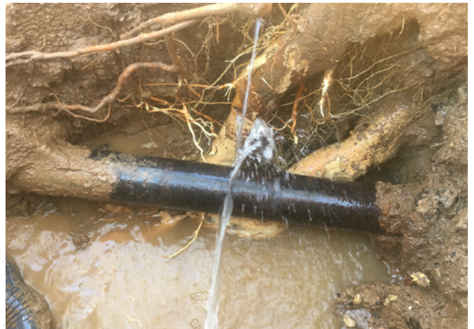
Close up on impact of tree root causing lateral pressure on a 100mm cast iron water main.
