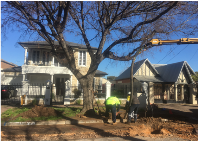
Tree planted less than 1 metre from water main.
