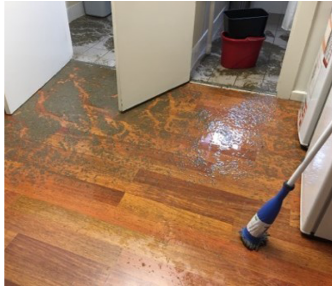
An example of a customer internal wastewater overflow.
