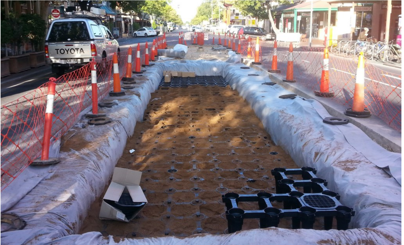
Gouger Street tree planting trial using strataCells installed in preparation for tree planting.
