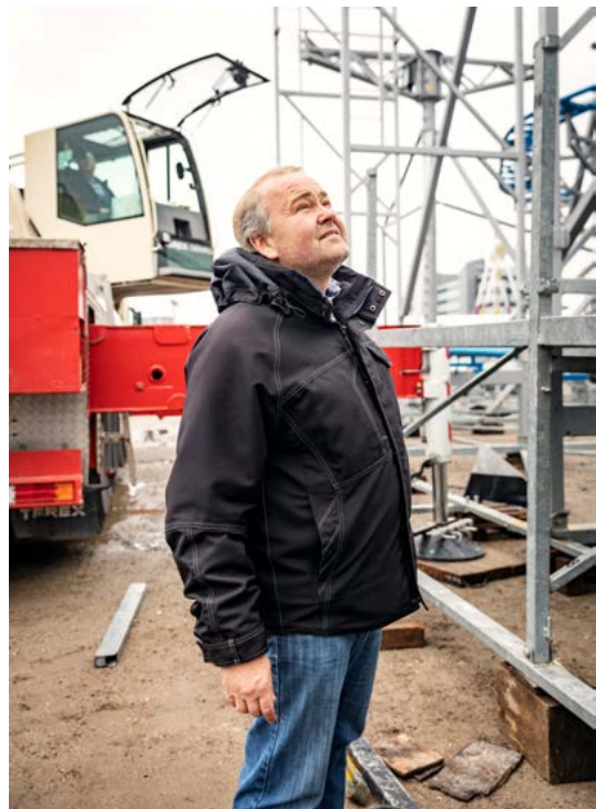
The boss, Mike Ahrend, supervises the installation and directs his ten workers
