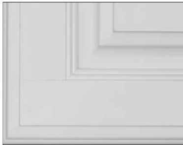
Example of front joint separation
