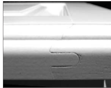
Example of end joint separation
