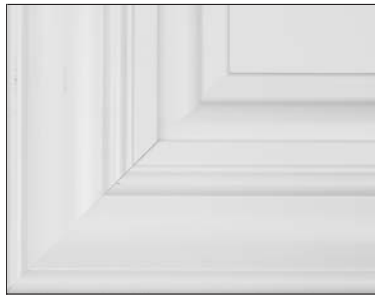
Example of front joint separation
