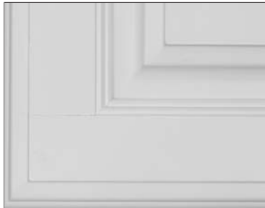
Example of front joint separation
