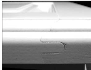
Example of end joint separation
