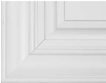
Example of front joint separation
