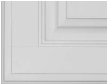
Example of front joint separation
