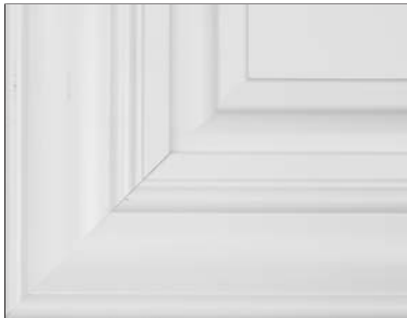
Example of front joint separation
