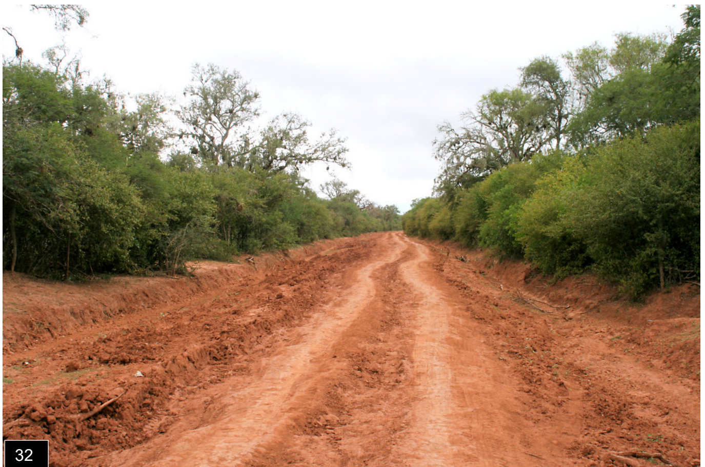
Fig. 32: During rainfall the roads in locality 5 become impassable
