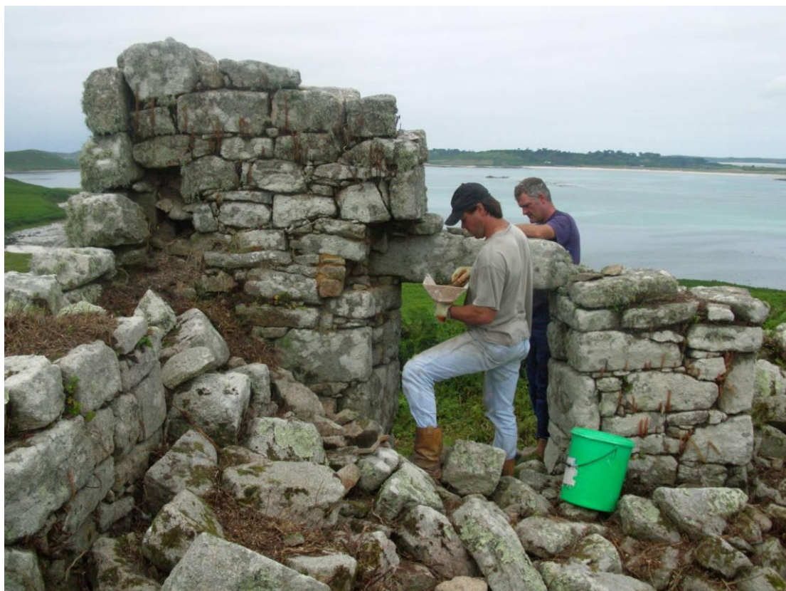
Fig 9.6 Consolidation work being carried out on House N on Samson in July 2006 (photo:Jacqui Mulville)
