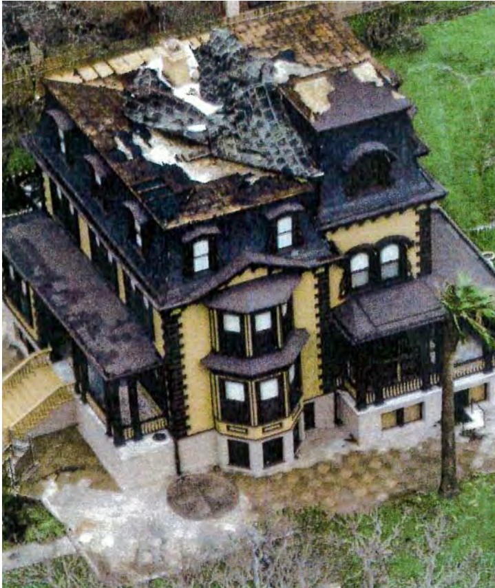
Aug. 2017: Fulton Mansion State Historical Site, damage from Hurricane Harvey (photo courtesy of Fulton Mansion Education and History Center)
