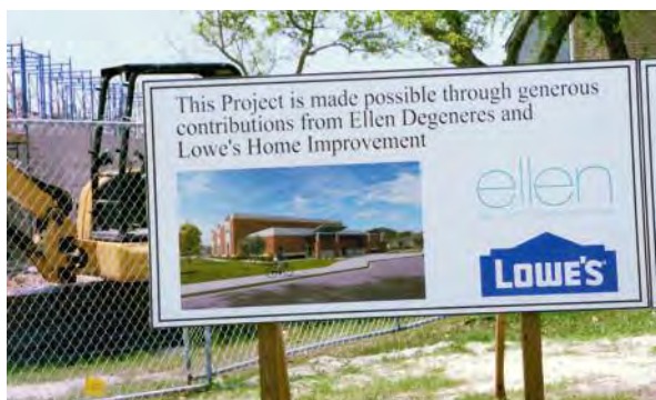
Aug. 2019: The new high school gym under construction. Thank you, Ellen Degeneres and Lowes.
